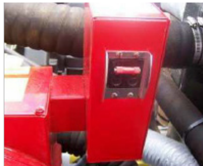
Power switch that activates electricity
