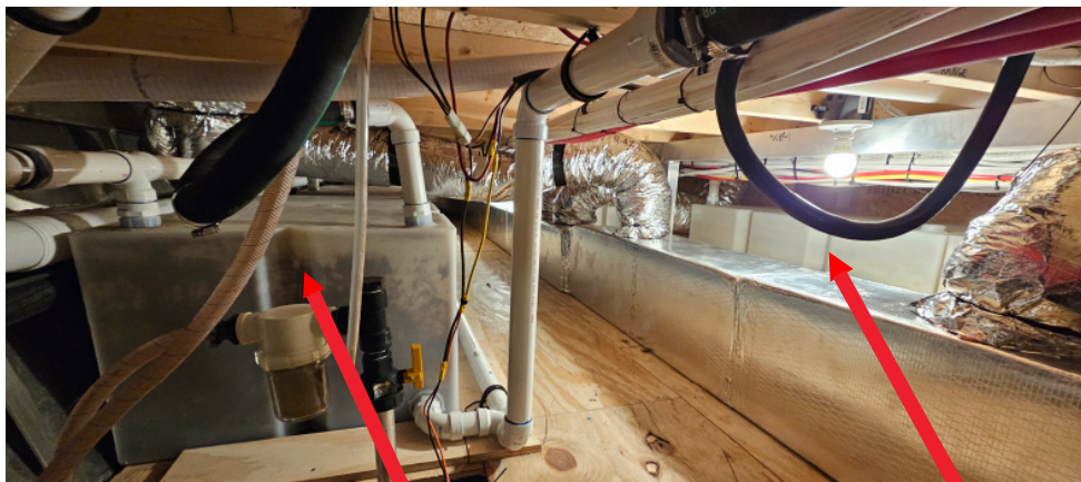
Black Water Tank
