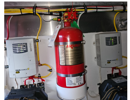
Fire Suppression System
