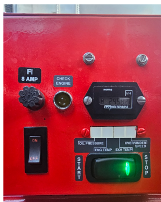
Generator "ON" switch and starter
